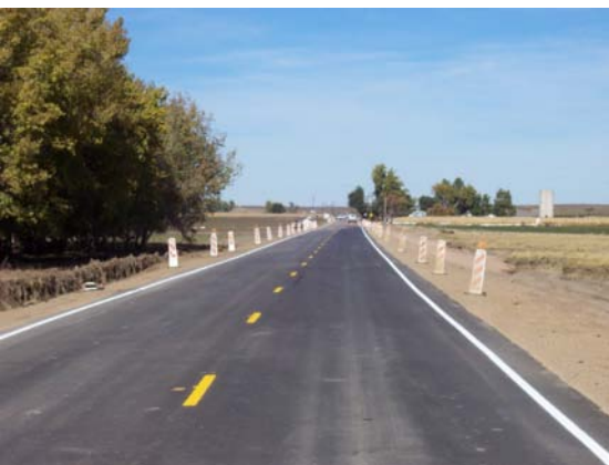
Weld County Road 61 after the flood (left) and after temporary repairs (right) were completed earlier this week. (Photos courtesy of Weld County.)
