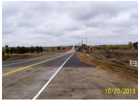
Flood waters not only destroyed a large portion of Weld County Road 13 but also utility lines (left). Temporary repairs on the road mean travelers can once again use the road but are cautioned to be mindful of the new reduced speed limit. (Photos courtesy of Weld County.)
