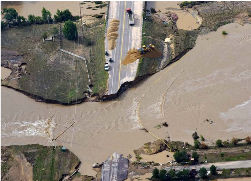
Weld County Road 13 sustained major damage in the September flood. Rushing waters carved a 300' wide path through the road and destroyed water, gas and sewer lines. (Photo courtesy of Weld County.)
